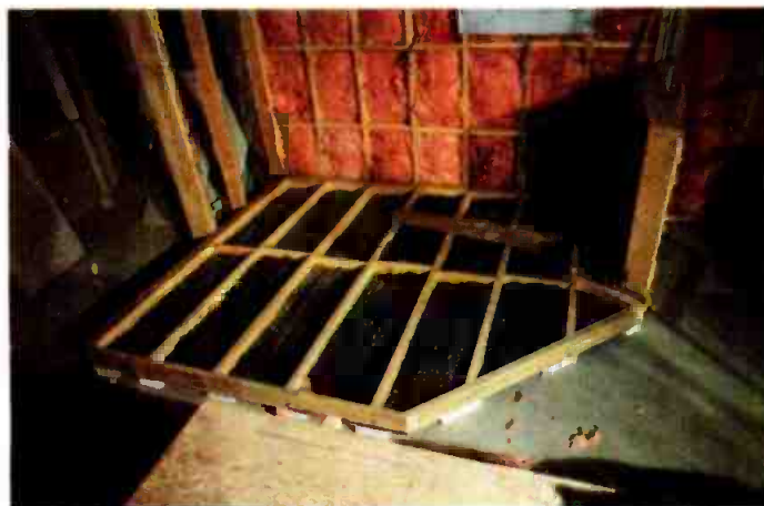
Starting the drum booth showing the sand drying out and styrofoam strips underneath.
