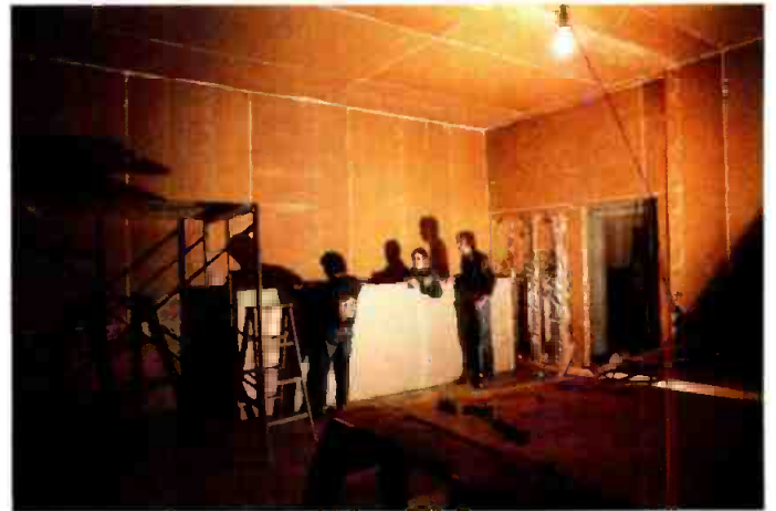
Starting to hang gypsum over sound deadening board on resilient channel in control room, showing caulking on seams.
