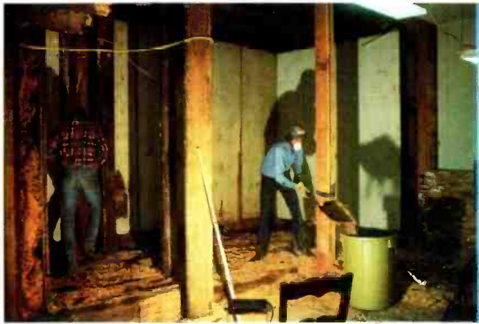
Removing sawdust insulation from old floor in future location of control room.
